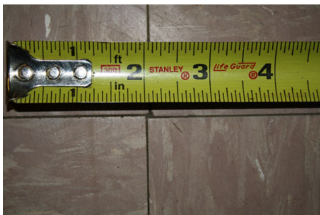
Photo 3: VCT run off and gaps at joints.
